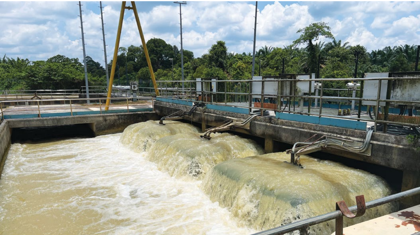
Raw water transfer pump from Sungai Johor to Upper Layang Dam, Sg Layang, Pasir Gudang, with a capacity of 180 million liters per day
